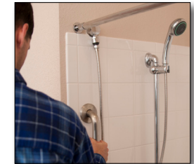
We install grab bars for safety.
