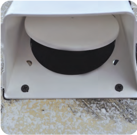
5. Termination has backdraft damper and no cage
