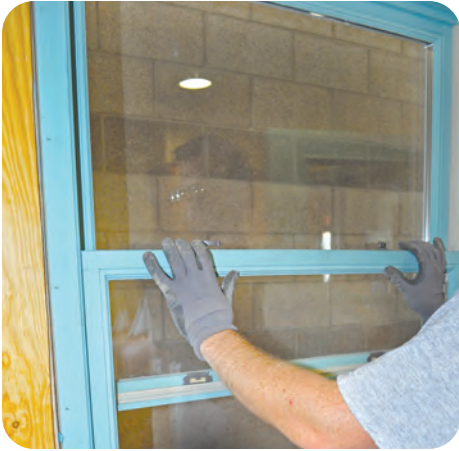
7. Ensure window is operational
