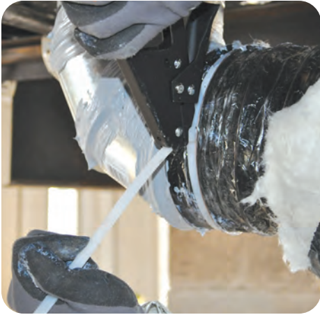
1. Secure duct liner to hard connections with zip tie and tensioner tool
