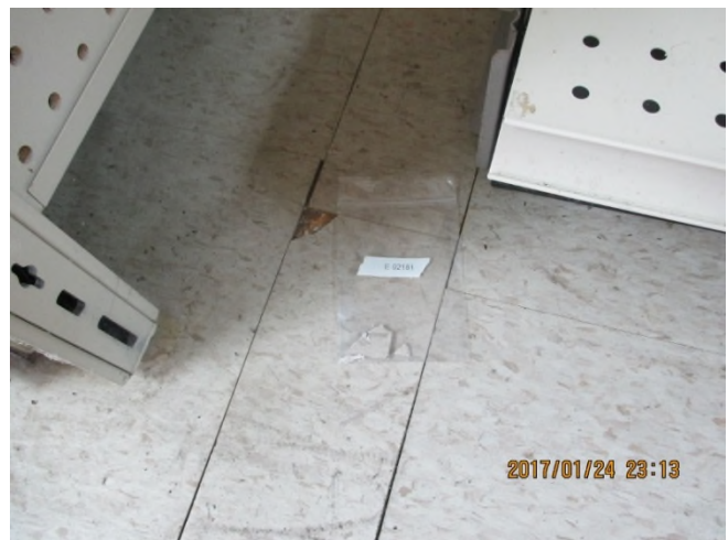
Photo 6: View of tan VFT and associated mastic sample location.
