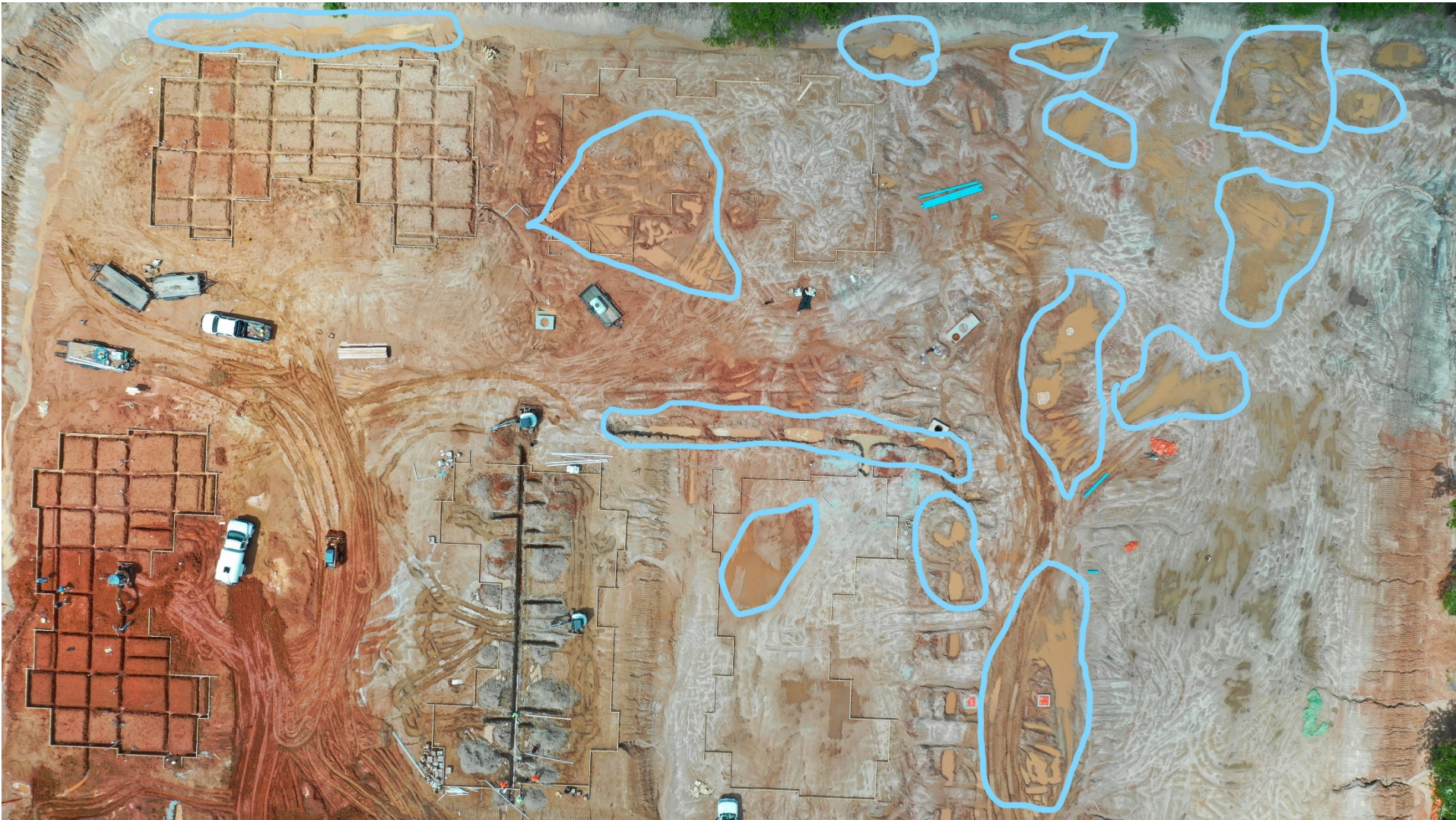
Rain –Standing water in blue circles. Workers trying to pump water out of work area.
