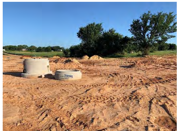
Photo 6: Final sanitary sewer manhole installation to be completed at west side of site.
