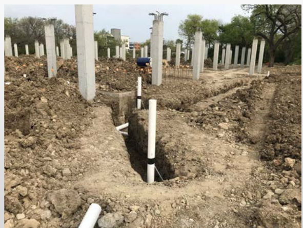
Plumbing at Building B
