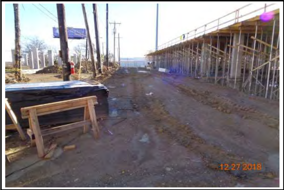
Photograph 2: Muddy site conditions at Building "A".
