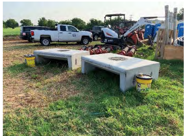
Photo 12: Stocked stormwater curb inlets.
