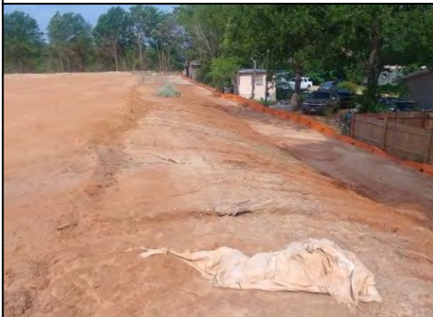
Photo # 9 Building 1 - Contractor is contemplating install of retaining wall near the bottom of slope
