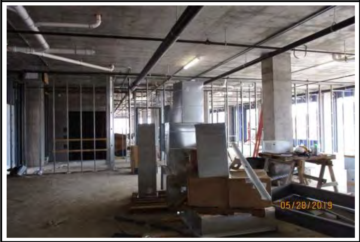
Photograph 3: Metal stud framing in medical clinic on first floor at Building "A".
