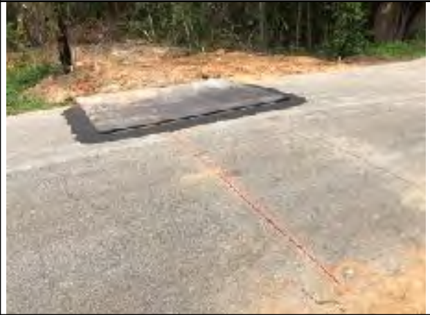
Photo # 2 Sanitary sewer connection at Lindale Cemetery Road
