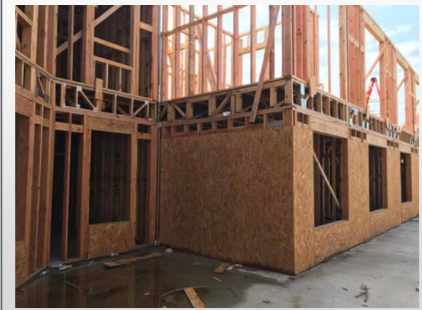
Move window per RFI at Firewall location
