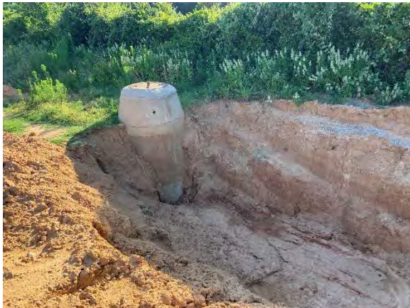
Photo 9: Completed sanitary sewer tie-in to existing manhole at east side of site.
