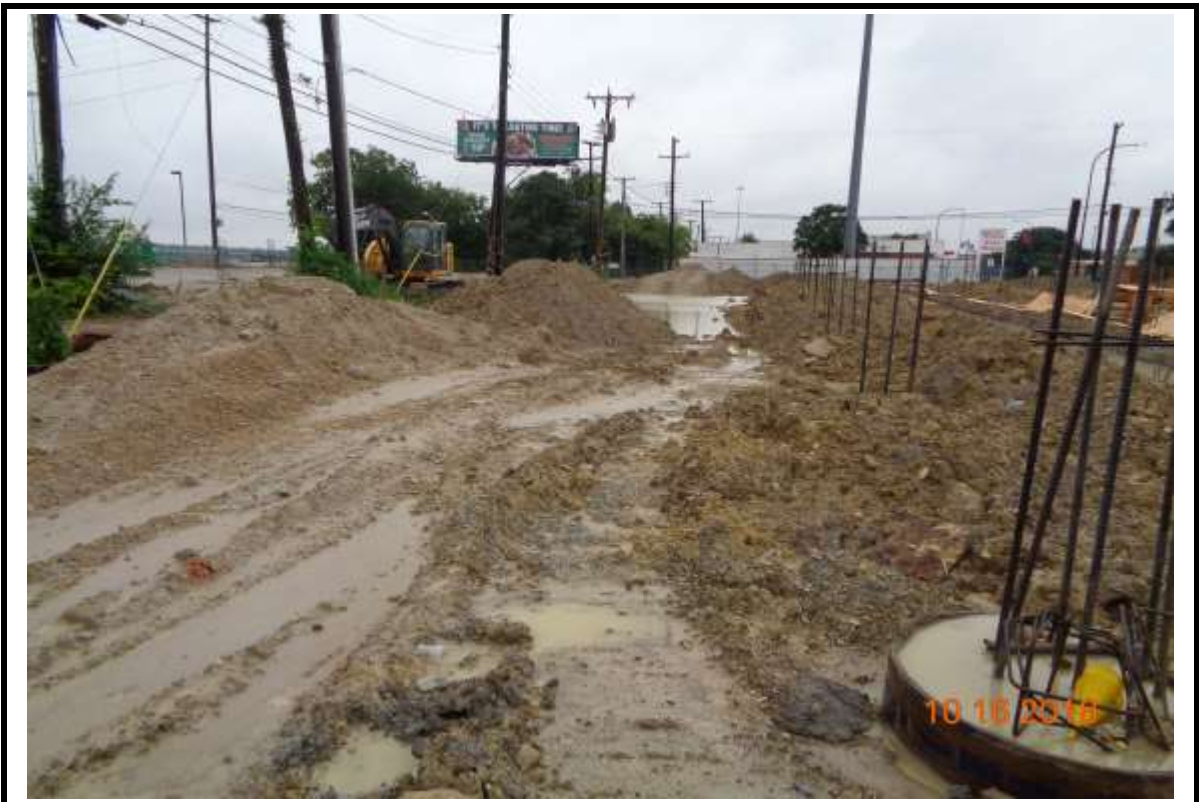
Photograph 4: Access way between Buildings "A" and "B". Note drilled piers in place.
