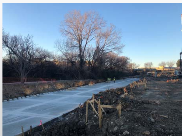
Building A fire lane concrete being placed, ongoing progress of fire lane
