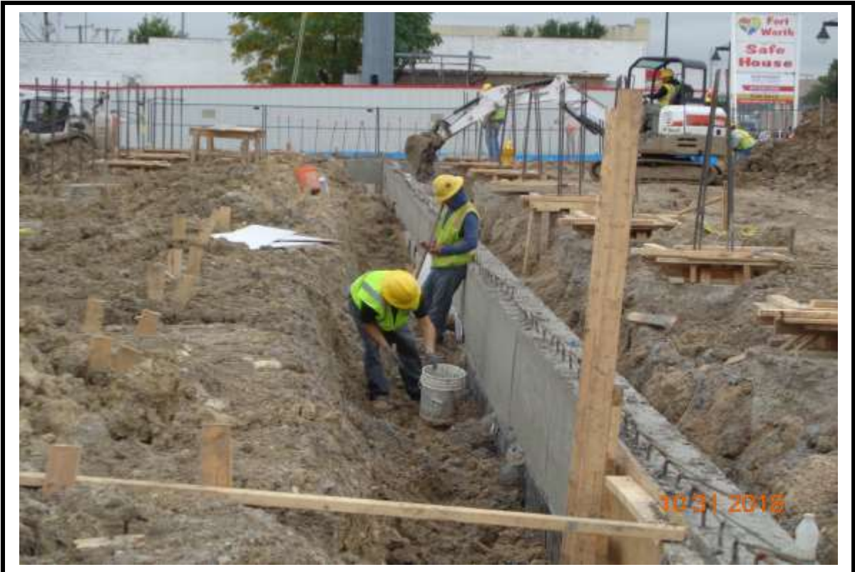
Photograph 10: Rubbing form tie holes at North beam Building “A”.
