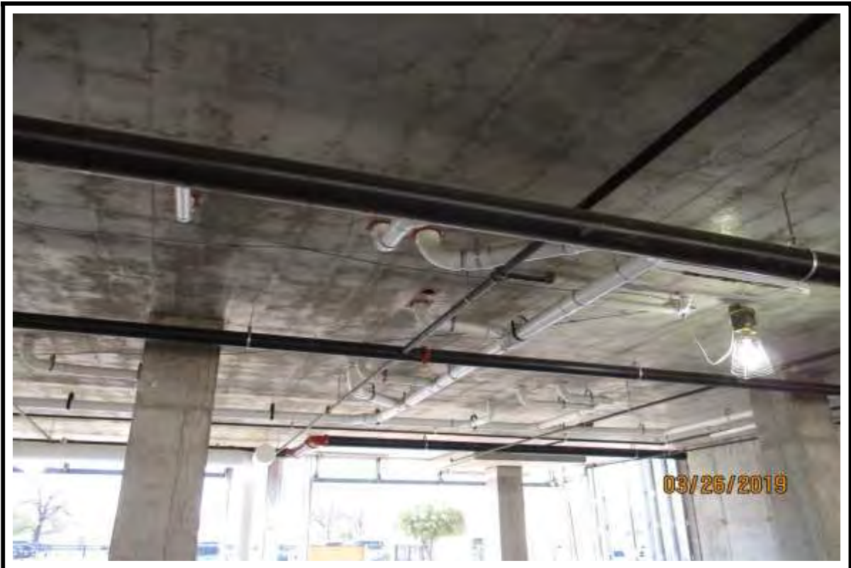
Photograph 6: Fire sprinkler piping at Building "A".
