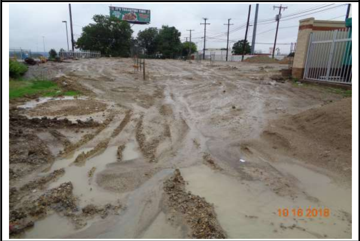
Photograph 3: Building pad at Building "B". Site is very wet from recent rains.
