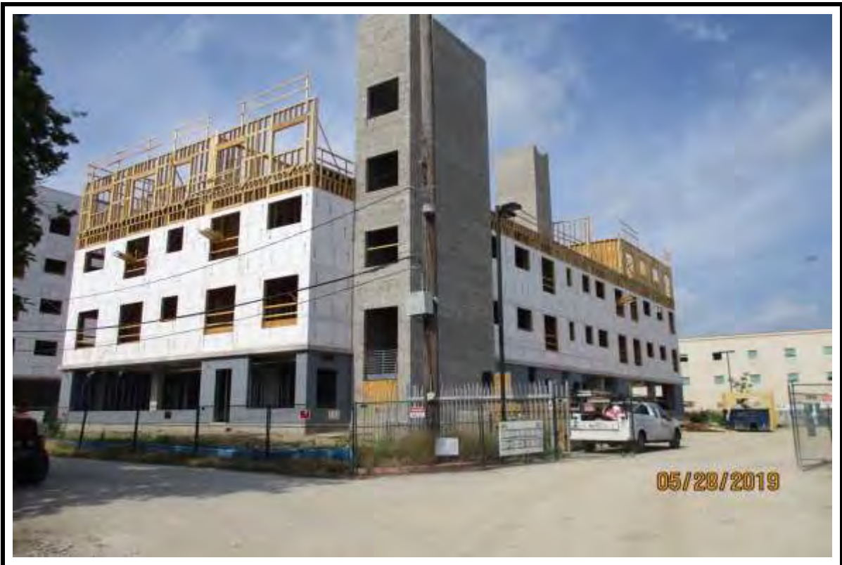
Photograph 6: CMU stair towers and wood framing to 4 th floor at Building "B".
