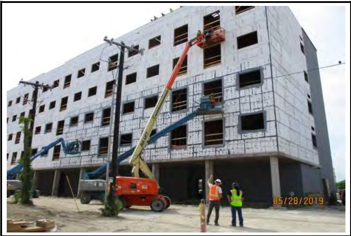
Photograph 1: Sealing exterior sheathing joints and screw heads prior to exterior finishes at Building "A".
