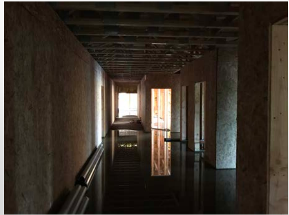
Standing water at unit framing above podium
