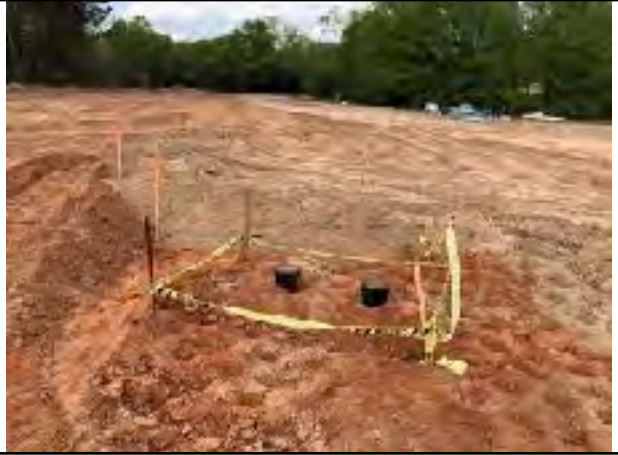
Photo # 8 Detail of installed water valves
