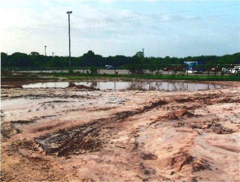
Status of detention pond on the West side of the property.
