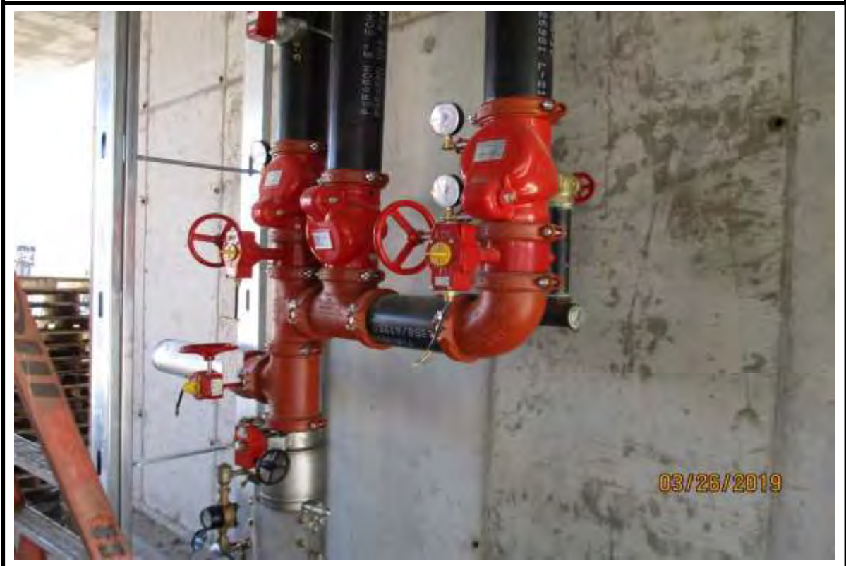
Photograph 7: Main fire riser tree at Building "A".
