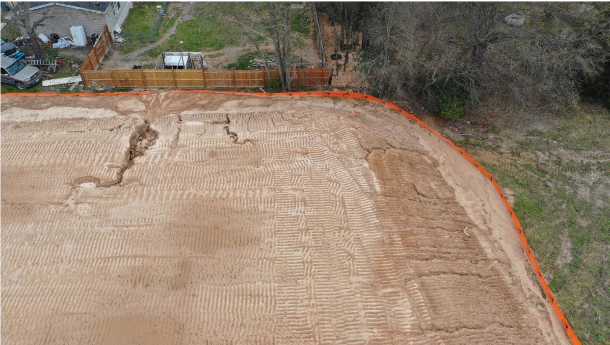
DJI130 –Building pad destroyed by abundant rain....must be rebuilt.
