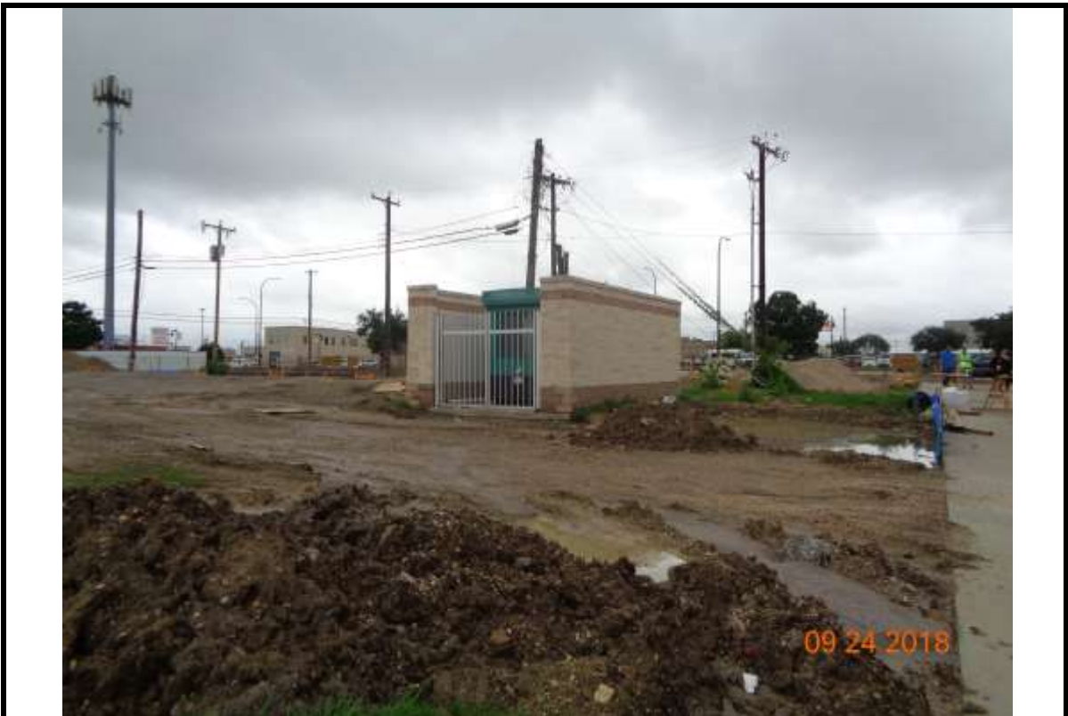
Photograph 10: Existing emergency generator on-site.
