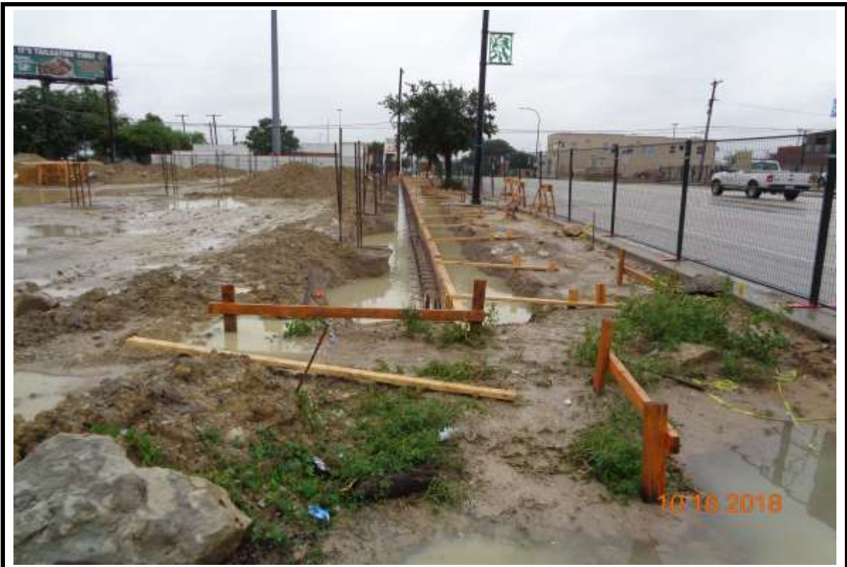
Photograph 6: North grade beam line at Building "A". Recent continuing rainfall is delaying the site work.
