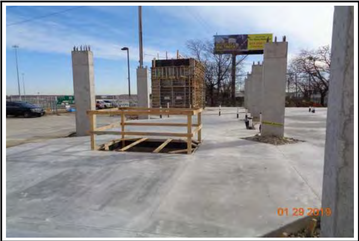
Photograph 4: Finished Common Area slab on grade with elevator pit at Building "B".
