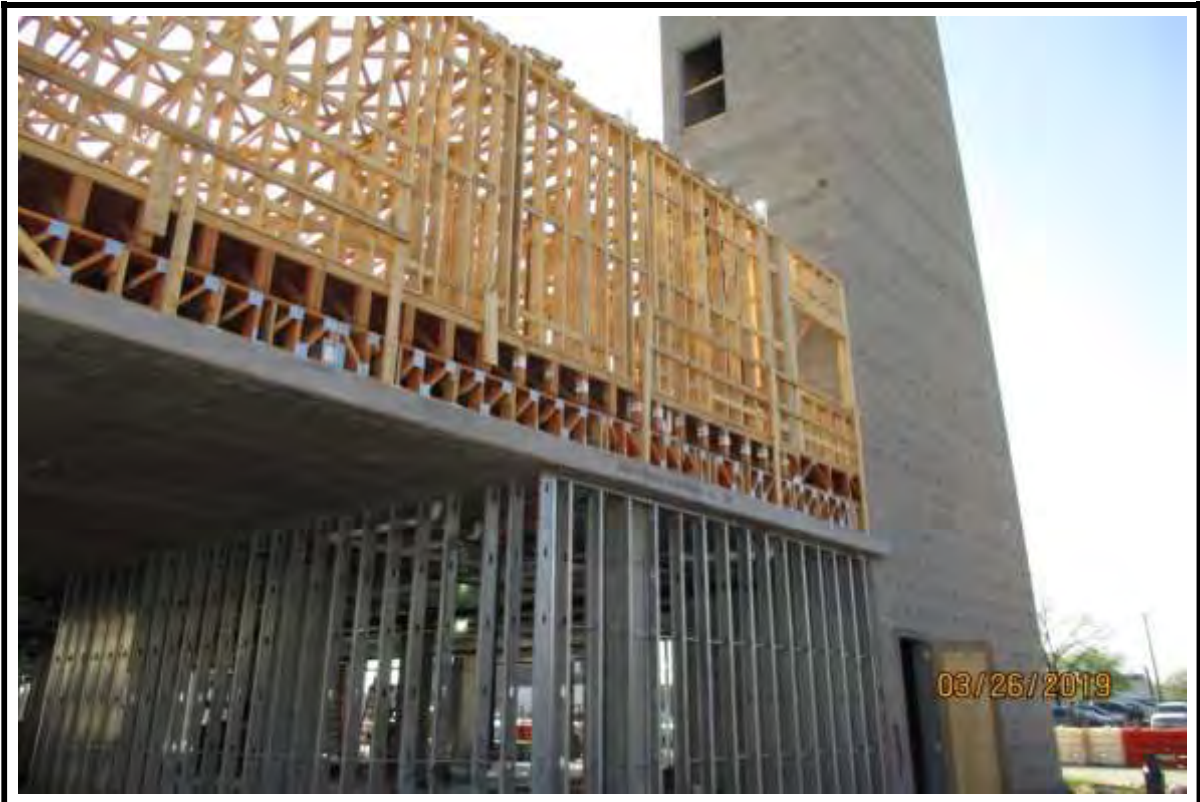
Photograph 1: 1 st floor metal wall framing with wood framing on podium above at Building "A".
