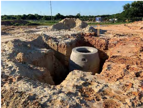
Photos 7 – 8: Sanitary sewer utilities and manhole installation at east side of site.
