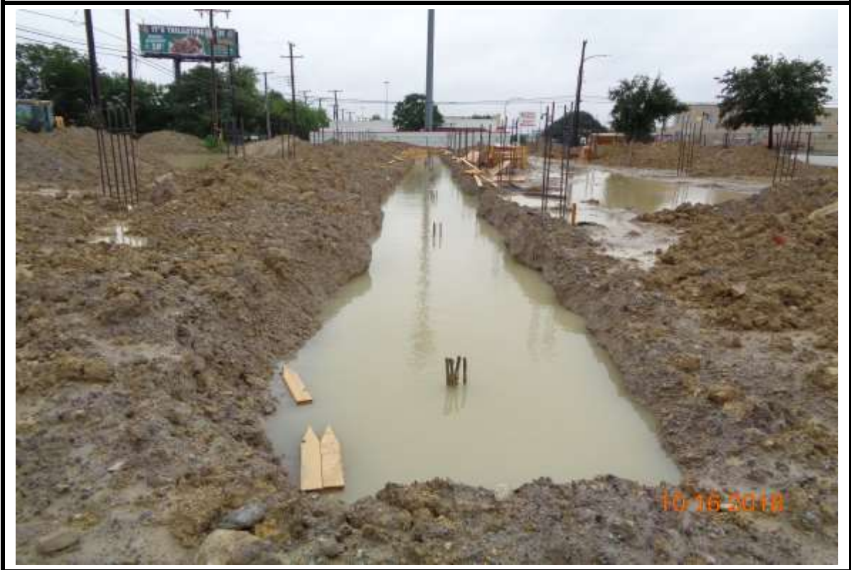
Photograph 5: South Grade Beam at Building "A". Recent continuing rainfall is delaying the site work.
