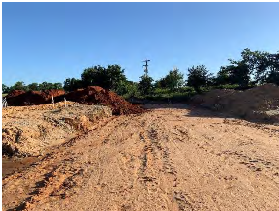
Photos 3 – 4: Earth fill and grading in progress for storm sewer culvert installation.
