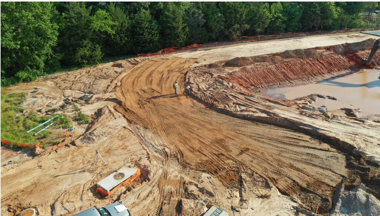
DJI202 -Entrance road being rebuilt after washing away to left side.
