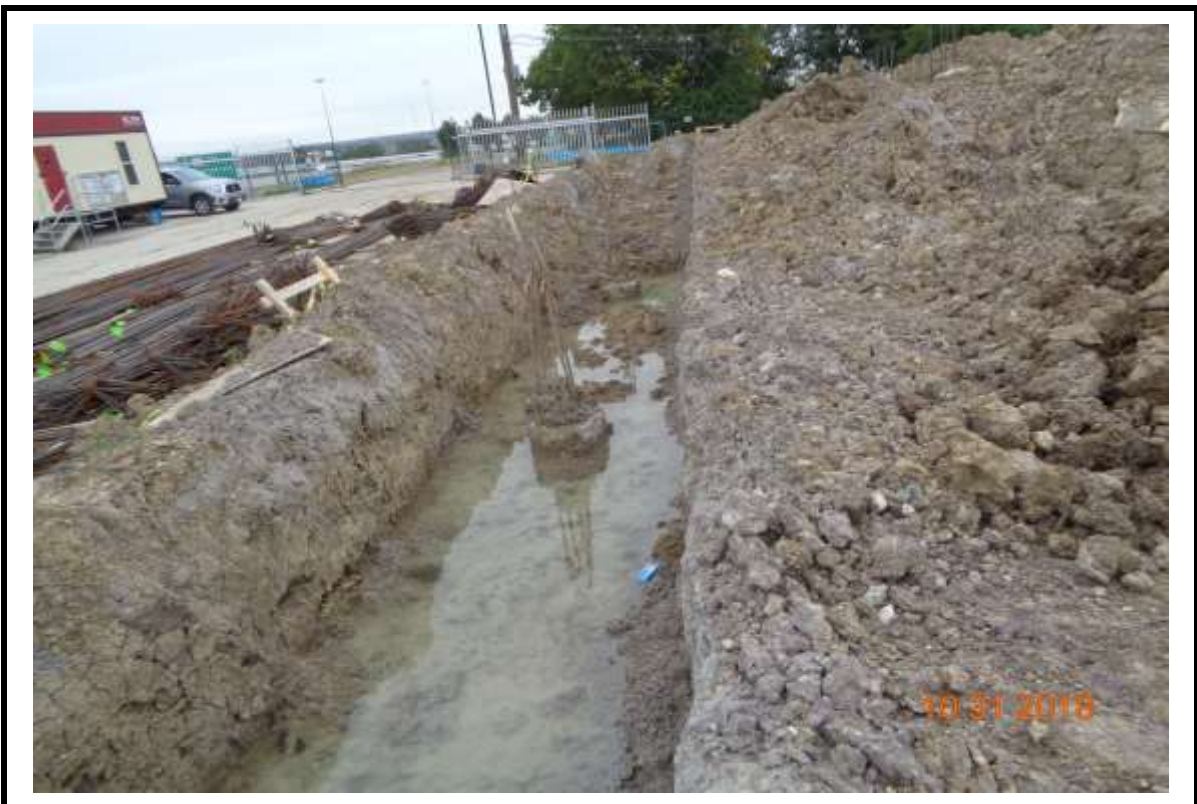
Photograph 2: Standing water at North grade beam excavation Building "B".
