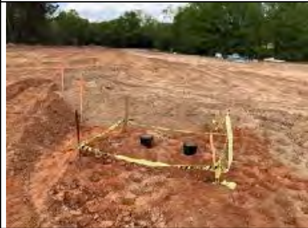
Photo # 9 Detail of installed water valves
