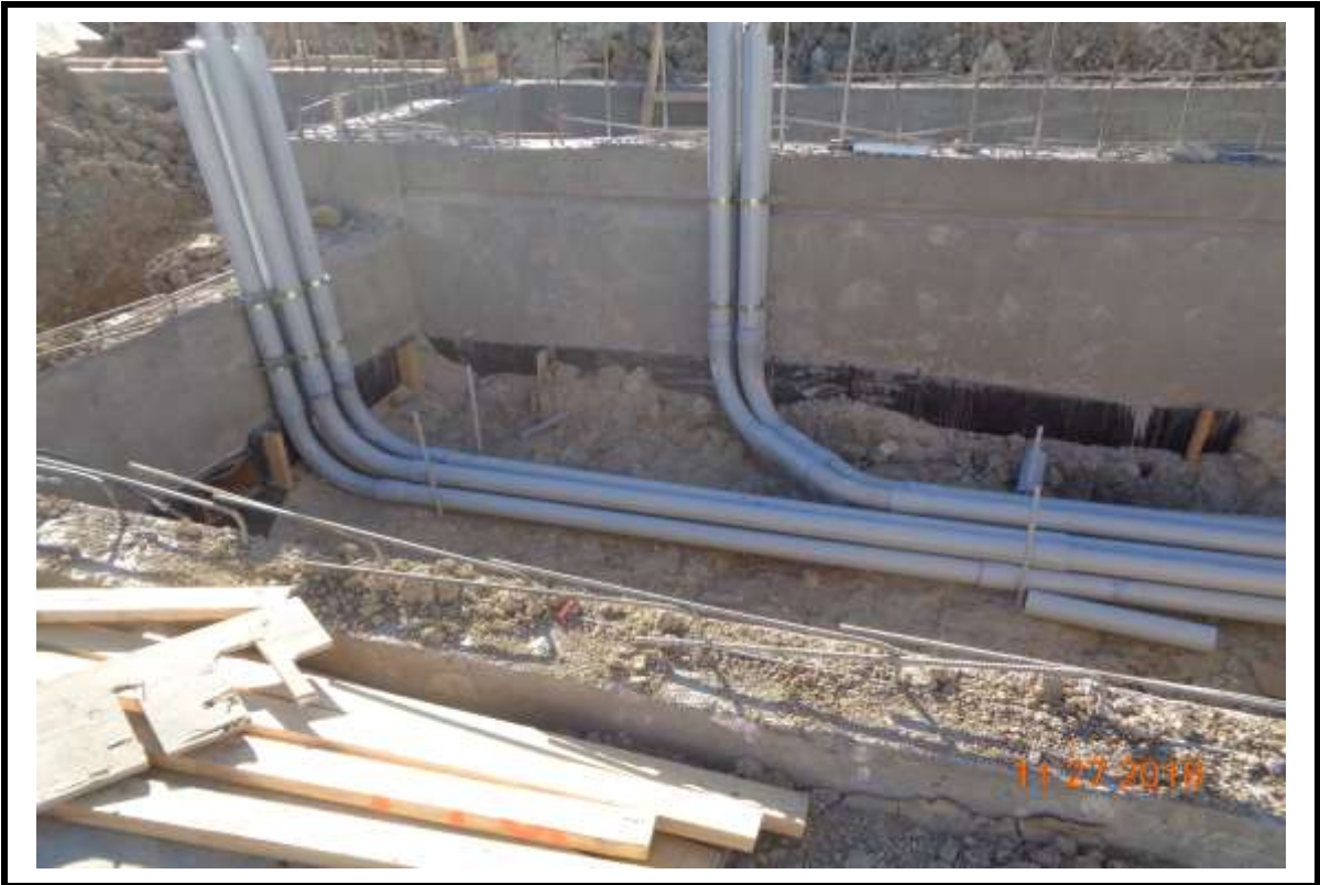
Photograph 4: Incoming electrical service conduits at Building “B”.
