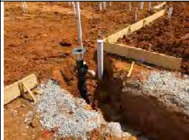
Photo # 15 Detail of fire water stub near building 6
