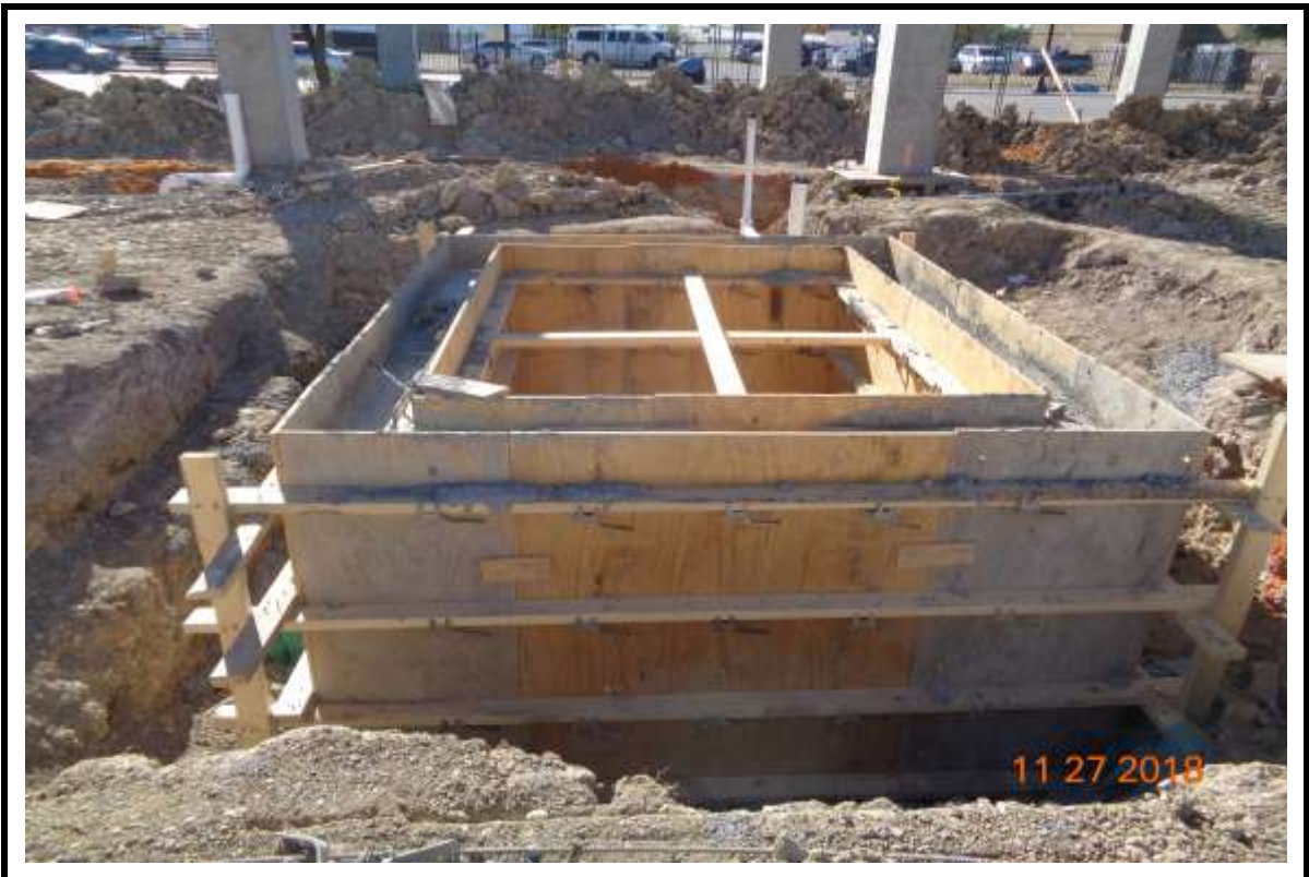
Photograph 8: Elevator pit at Building "A".
