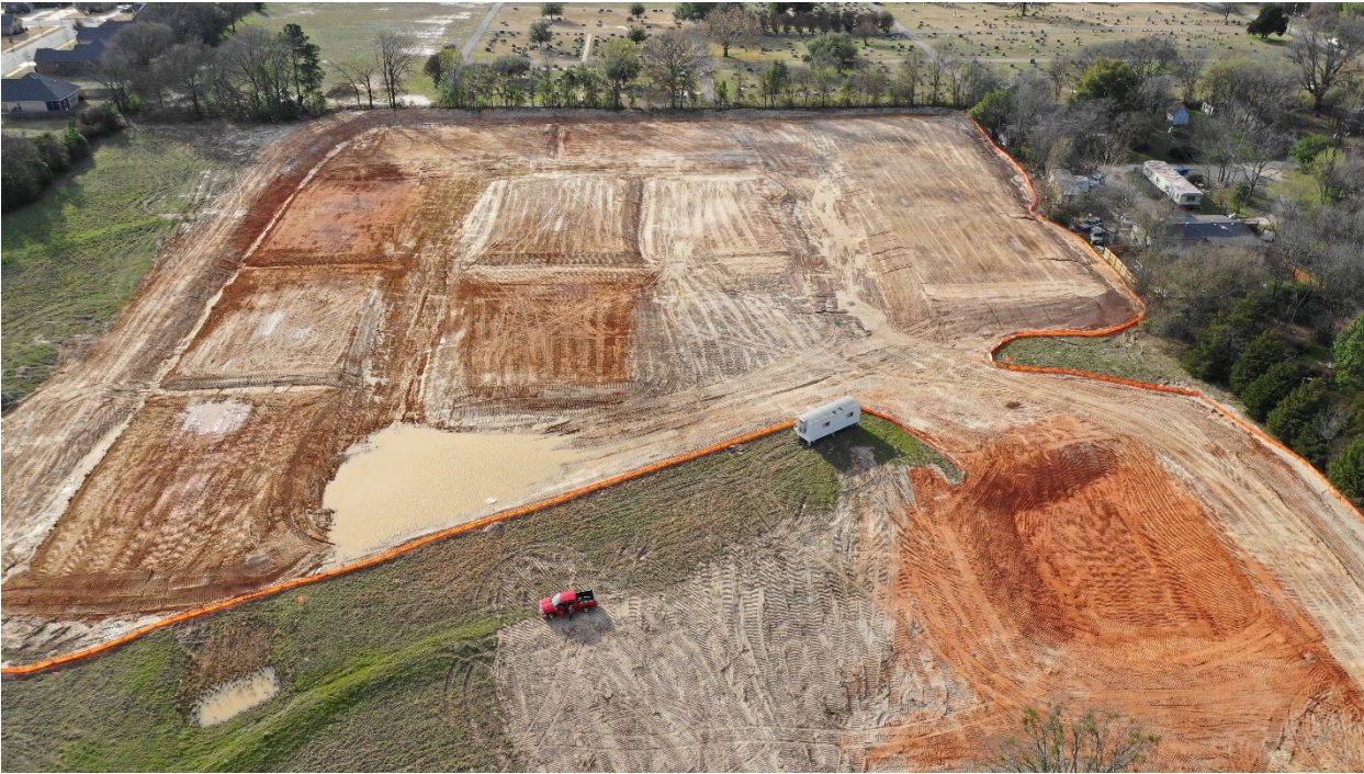
DJI128 –Water standing on site....work halted.
