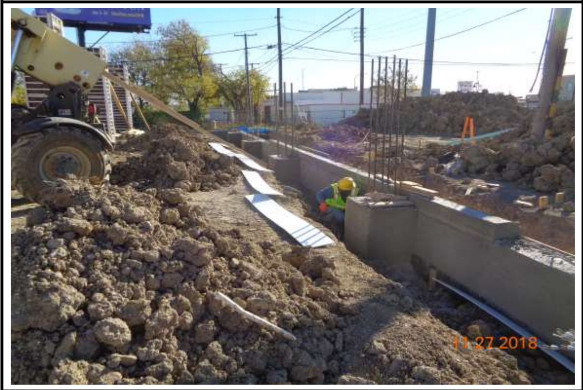
Photograph 5: Installing soil retainers at void boxes for grade beam at Building "A".
