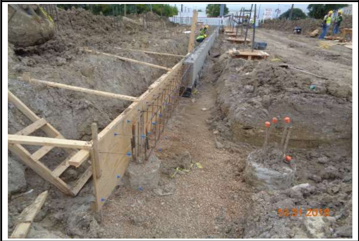
Photograph 5: Beam break at North grade beam Building "A".
