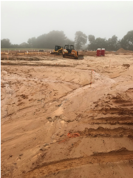
IMG158-All the roads and pads destroyed by heavy rains.
