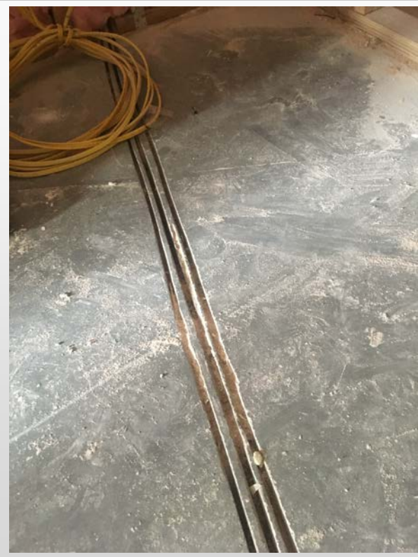
Building A – Ensure wire is in conduit
