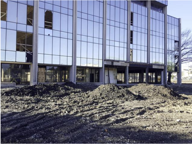
We visited the site on February 23, 2017. Existing Bank Building demolition was complete.
