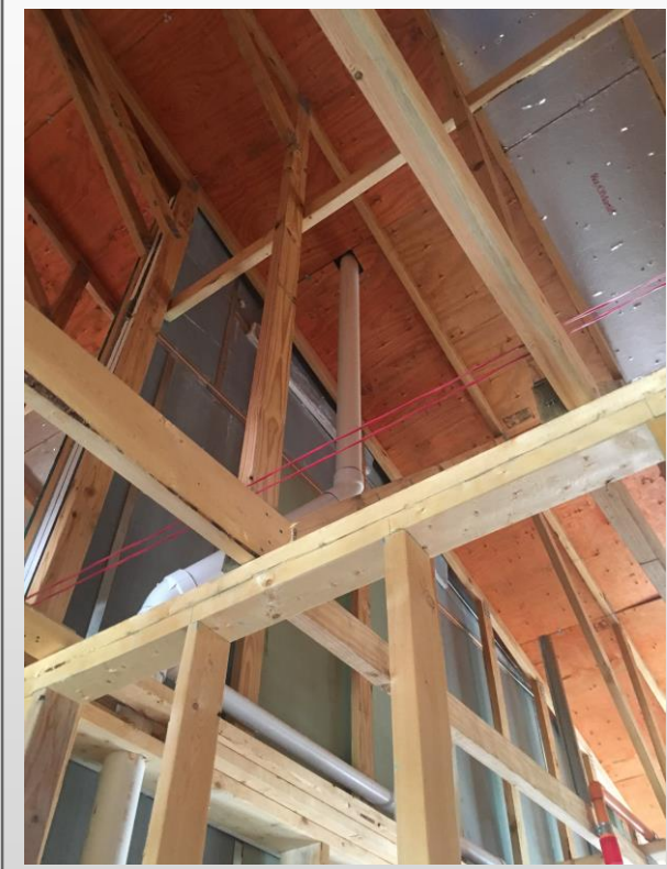
Plumbing within 4' of the firewall – needs to be relocated
