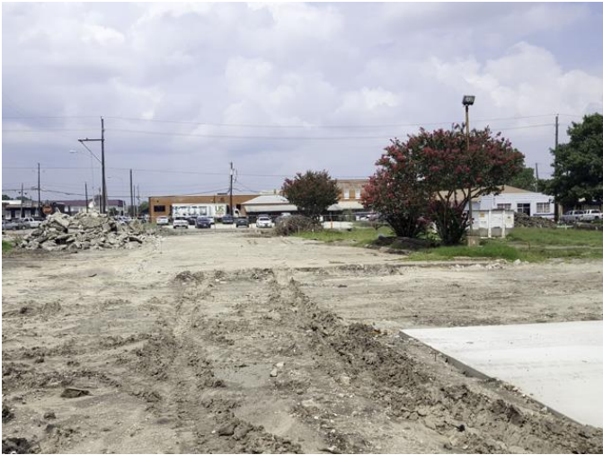
We visited the site on August 24, 2017. Existing site concrete paving demolition was complete.
