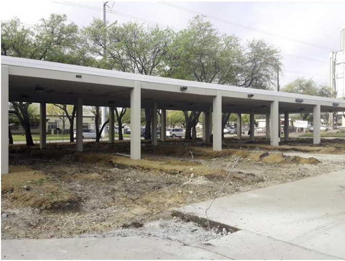
We visited the site on March 20, 2017. Existing site concrete paving demolition was substantially complete.
