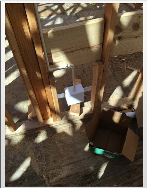
Building #1 non-rated boxes in rated walls to be wrapped or moved
