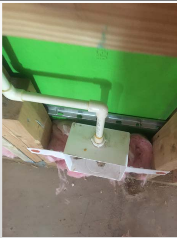
Building A – Ensure the non-rated boxes are putty packed
