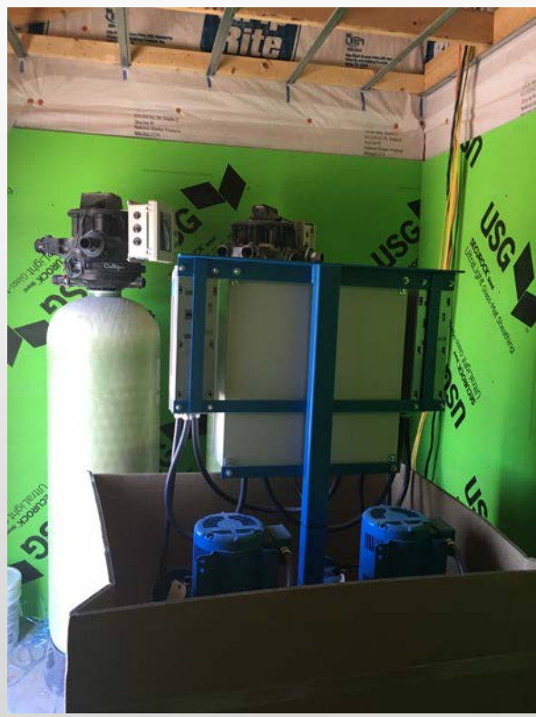
Building #2 Filtr Eq in place
