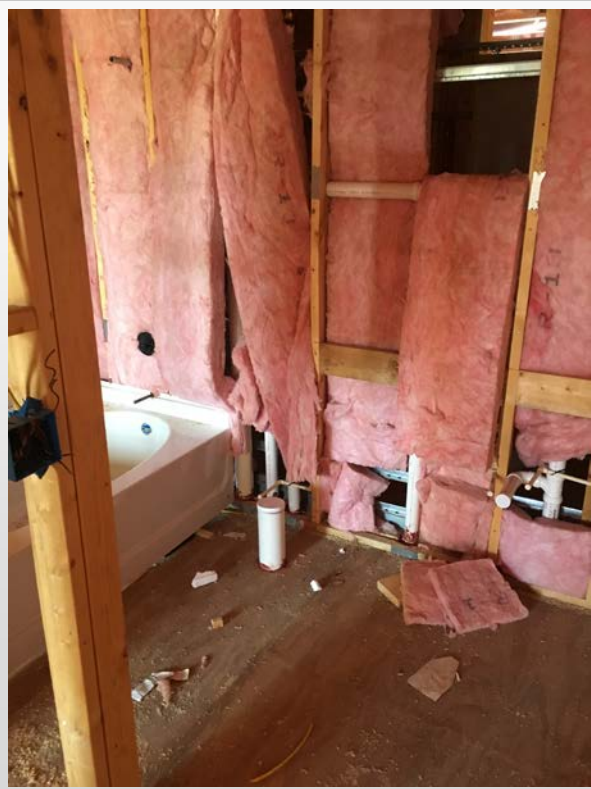
Building #2 ensure insulation is corrected before cover up
