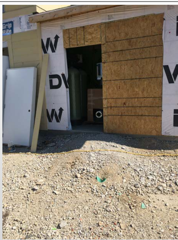
Building #2 Ensure missing building wrap is corrected prior to cover up
