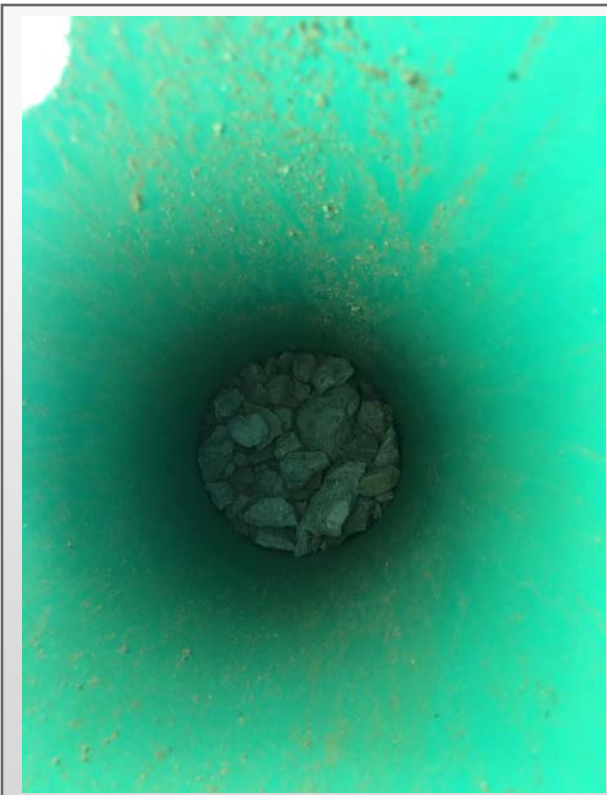
Building #2 Ensure cleanout pipes are clear prior to turnover
