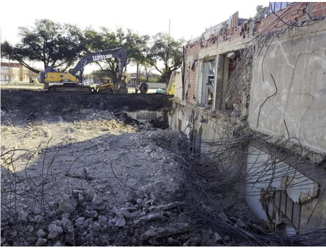
We visited the site on January 26, 2017. Existing Bank Building demolition was nearing completion.
