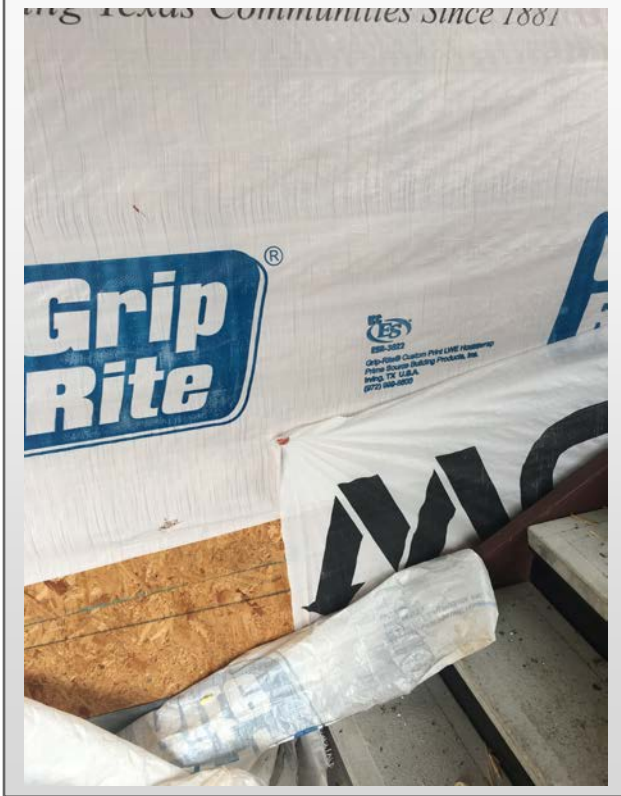
Building #2 stair tower WRB mis-lapped
