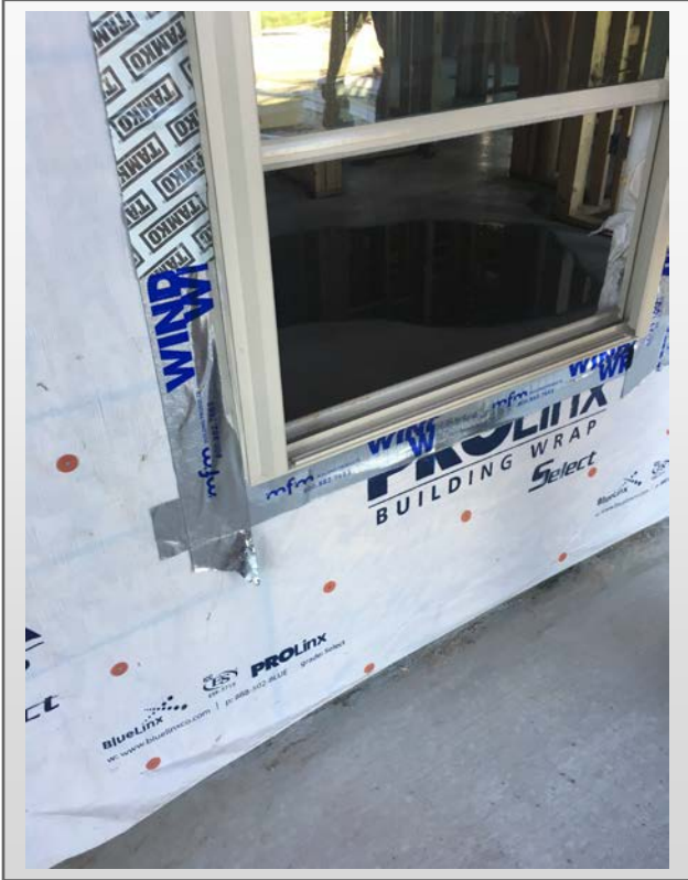
Building #1 building wrap and tape incorrectly installed
