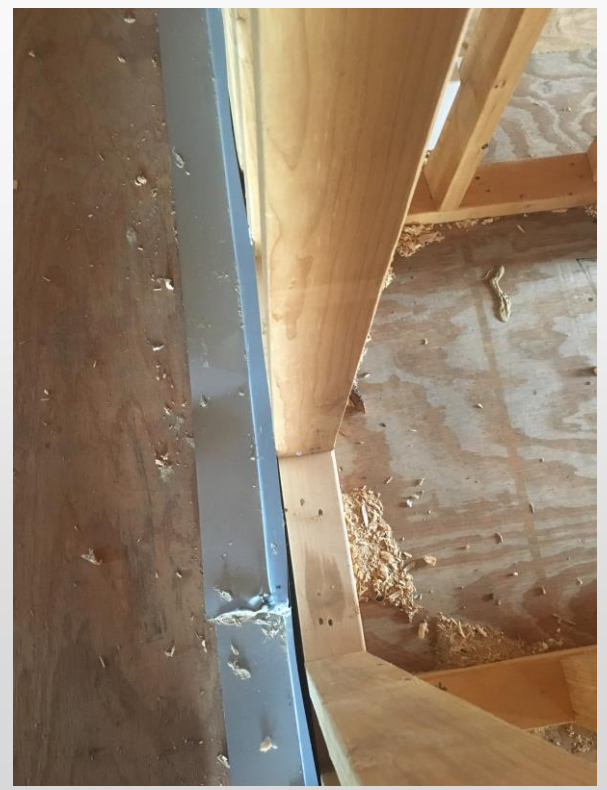
Breezeway flashing not tight to the wall – needs replacing
