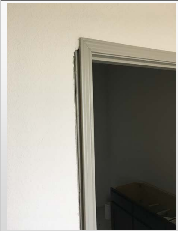
Building #1 trim at door leaves a gap
