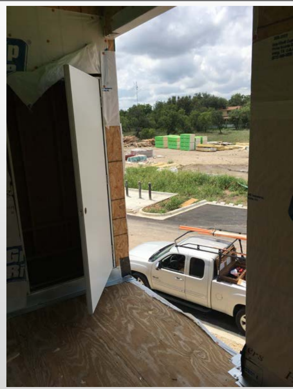
Building B - Missing some building wrap
