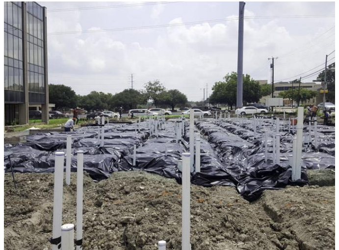
Building A under slab utility rough-ins were complete, with slab-on-grade reinforcing steel placement in progress.
