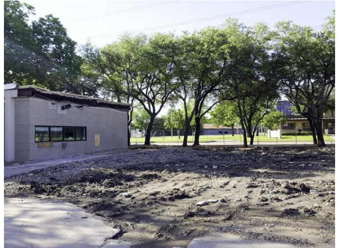
Existing drive-thru bank building demolition continued to be in progress and was nearing completion.
