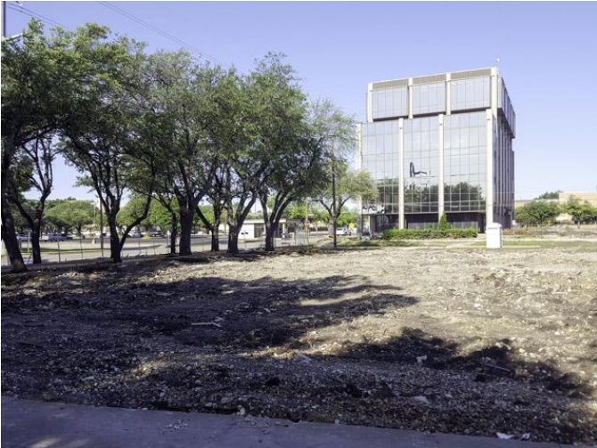
We visited the site on April 24, 2017. Existing drive-thru bank building demolition continued to be in progress and was nearing completion.
