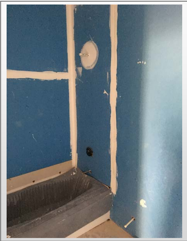
Building #1 – Typical tub needs code approved tile underlayment
