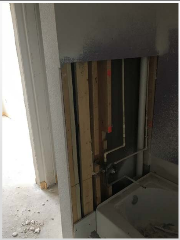
Building #1 tub wall extends too far
