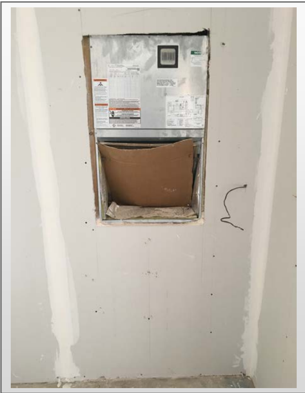
Building #1 typical HVAC needs access panel
