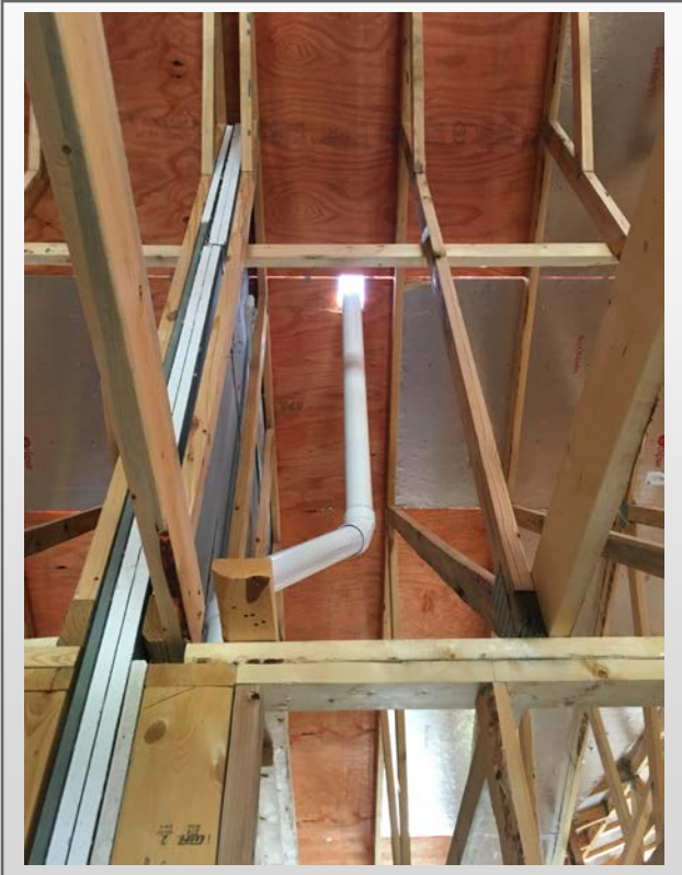
Building #2 firewall penetrations to be moved
