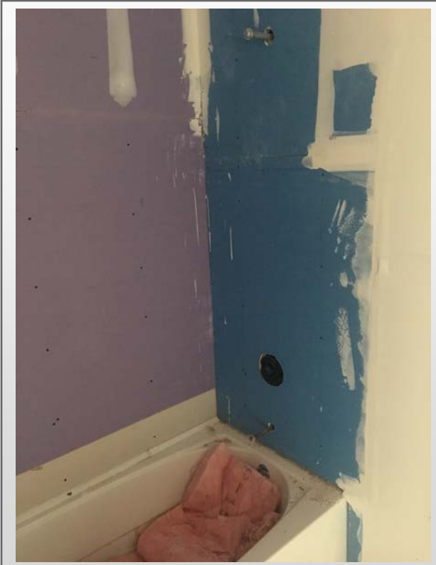
Building A – Ensure only Glass Mat is used behind the tub tile
