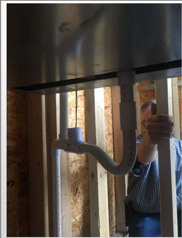
Building A – Ensure the overflow switch is installed per the MFG
