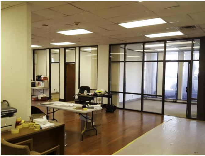
We visited the site on November 21 2016. Contractor was mobilized on-site within the existing building.
