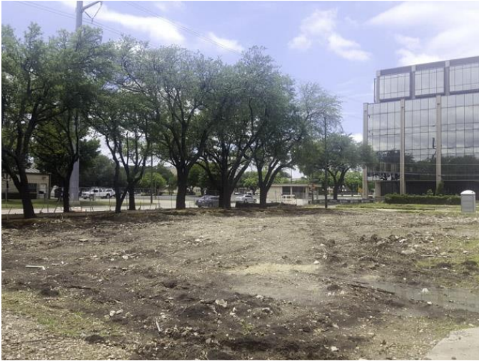
We visited the site on May 22, 2017. Existing drive-thru bank building and site demolition continued to be in progress and was nearing completion.
