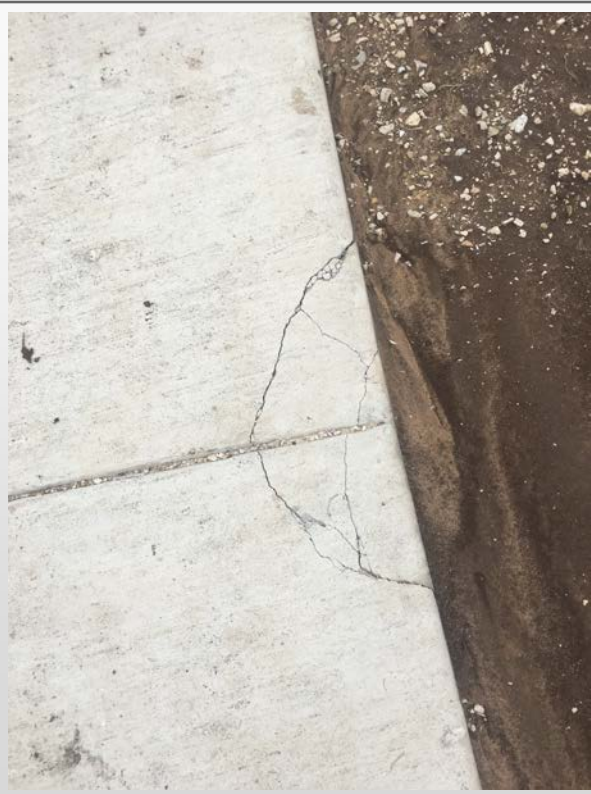
Misc. club sidewalk needing repair
